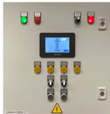
Hydraulics control panel
