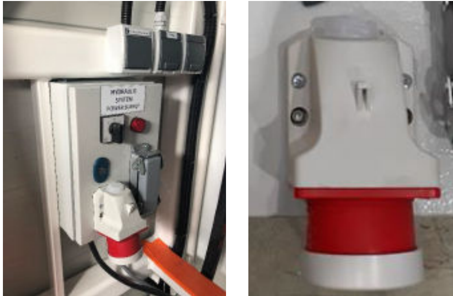
Figure 8 - The Hydraulic lifting system power connection
